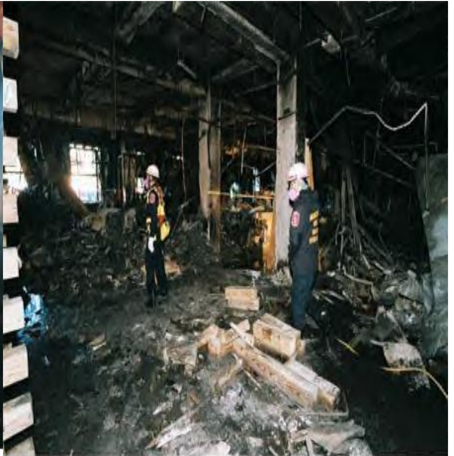
Arlington, VA, September 13, 2001 -- Urban Search and Rescue crews from Montgomery County work to clear debris and strengthen support at the crash site following Tuesday's attack.
