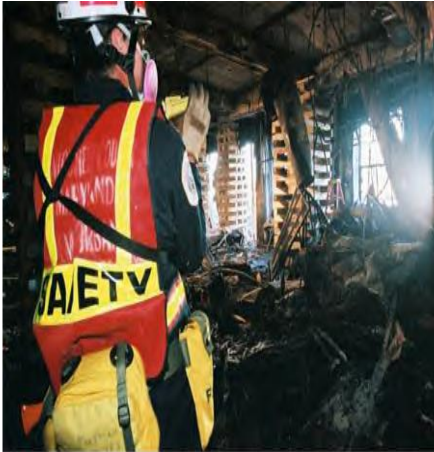
Arlington, VA, September 13, 2001 -- Urban Search and Rescue crews from Montgomery County work to clear debris and strengthen support at the crash site following Tuesday's attack.
